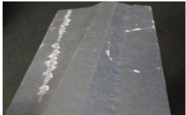
Note when scratched, the primer has been compromised as well as the presence of Zinc Oxide (white rust).
