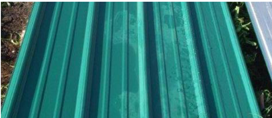
After just 3 months covered in the manner above, the panel bundle is opened to reveal that moisture has made its way into the layers of sheets.
