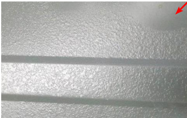
Close-up image of severe "Wet Stack Corrosion." Note smooth, normal surface in upper right corner.
