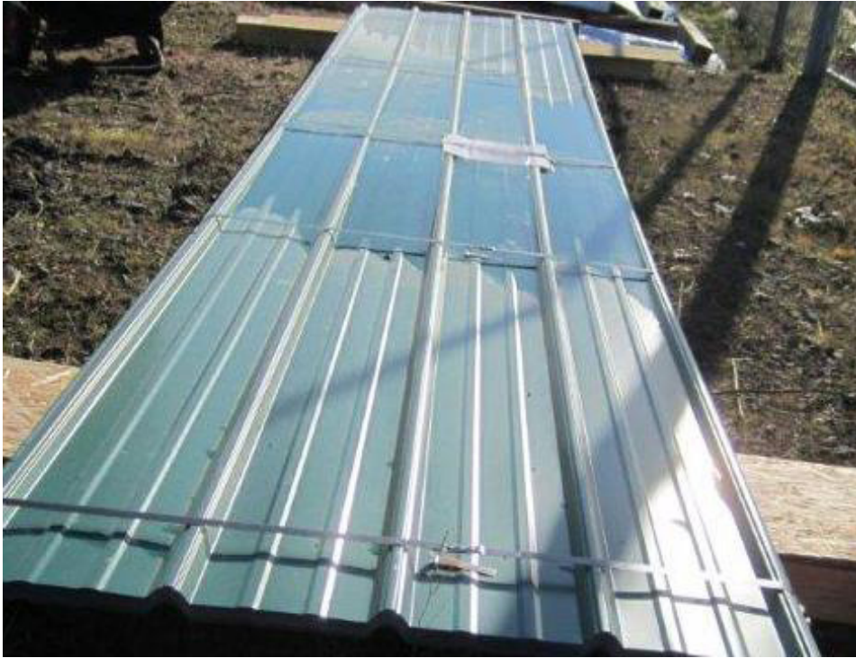
Insufficient support in the center of long panels allow "Bowling" or "Sagging" that traps water in the center of the panel length.
